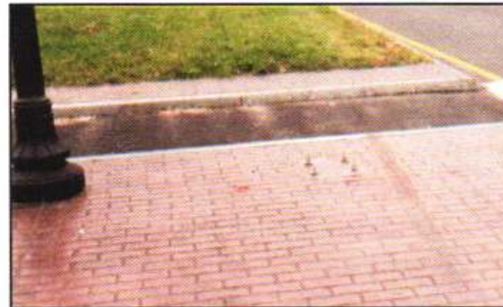
Figure 3.3.4.16: Evidence of a crash.
